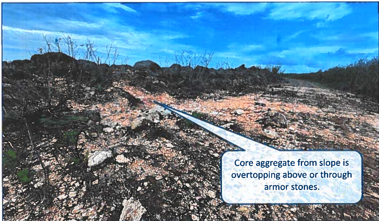
Photograph 4. Example of Debris Spills at Crest Road
